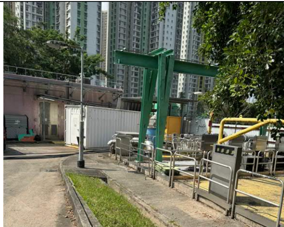
DSD Chung Yan Road Sewage Pumping Station
